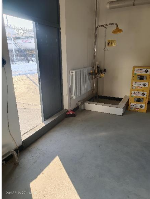
危化品危化试剂间围堰及防渗
