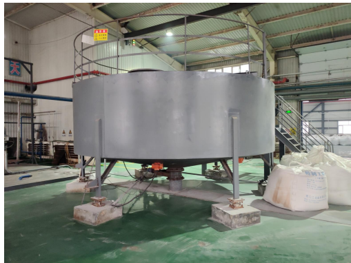
驱油型冲洗液投料槽
