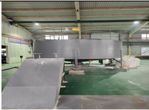
驱油型冲洗液投料槽
