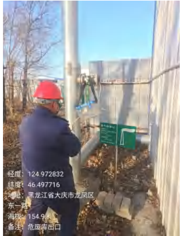
危废贮存库排气筒DA003
